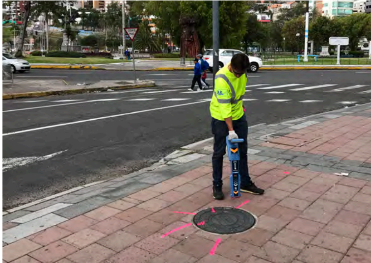
A professional SUE technician for SUE LATAM designates a line for the design phase of the Guayasamin project in Quito. As the first to use SUE in Quito, the project is a milestone for damage prevention in the nation.
